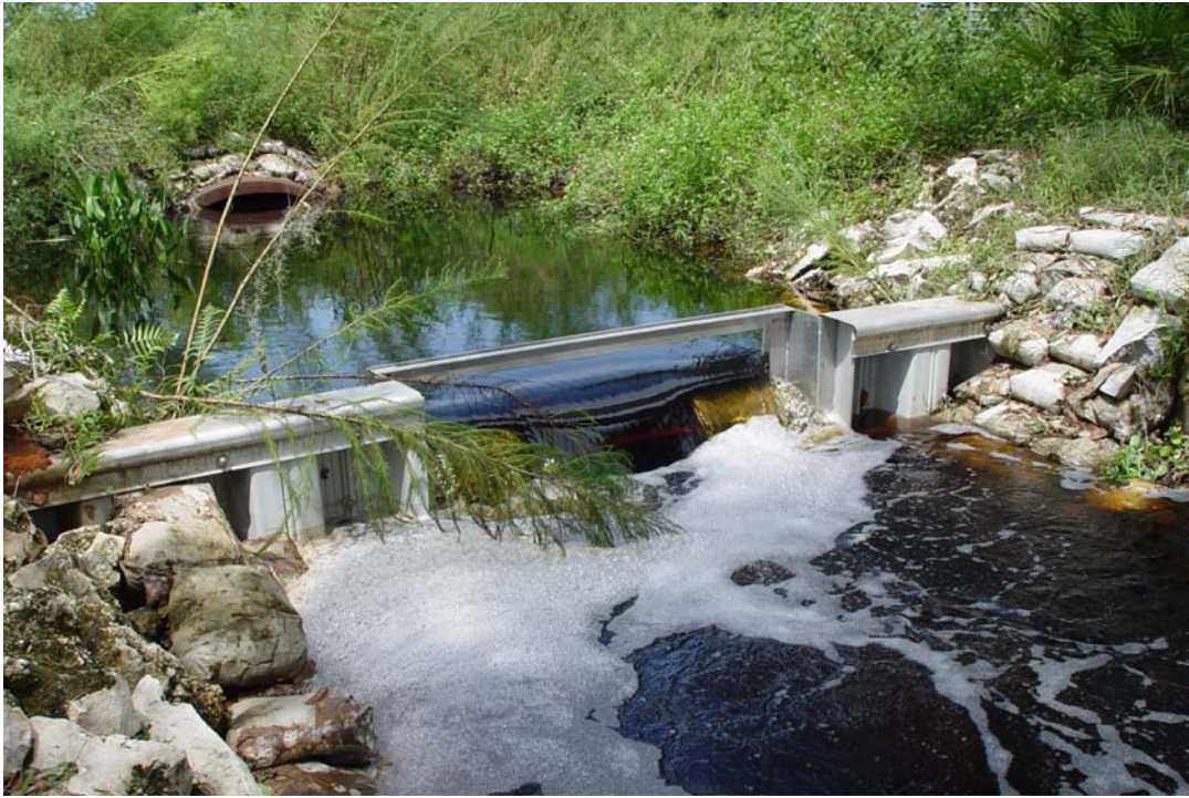
Photo 8. Flooding after Hurricane Jeanne in Sector C-5, at Weir C.
